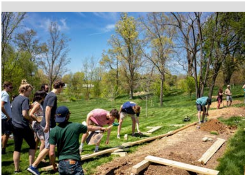
Students constructing pollinator garden beds on the East Campus Hillside. Photo by JMU Creative Media, Elise Trissel.
