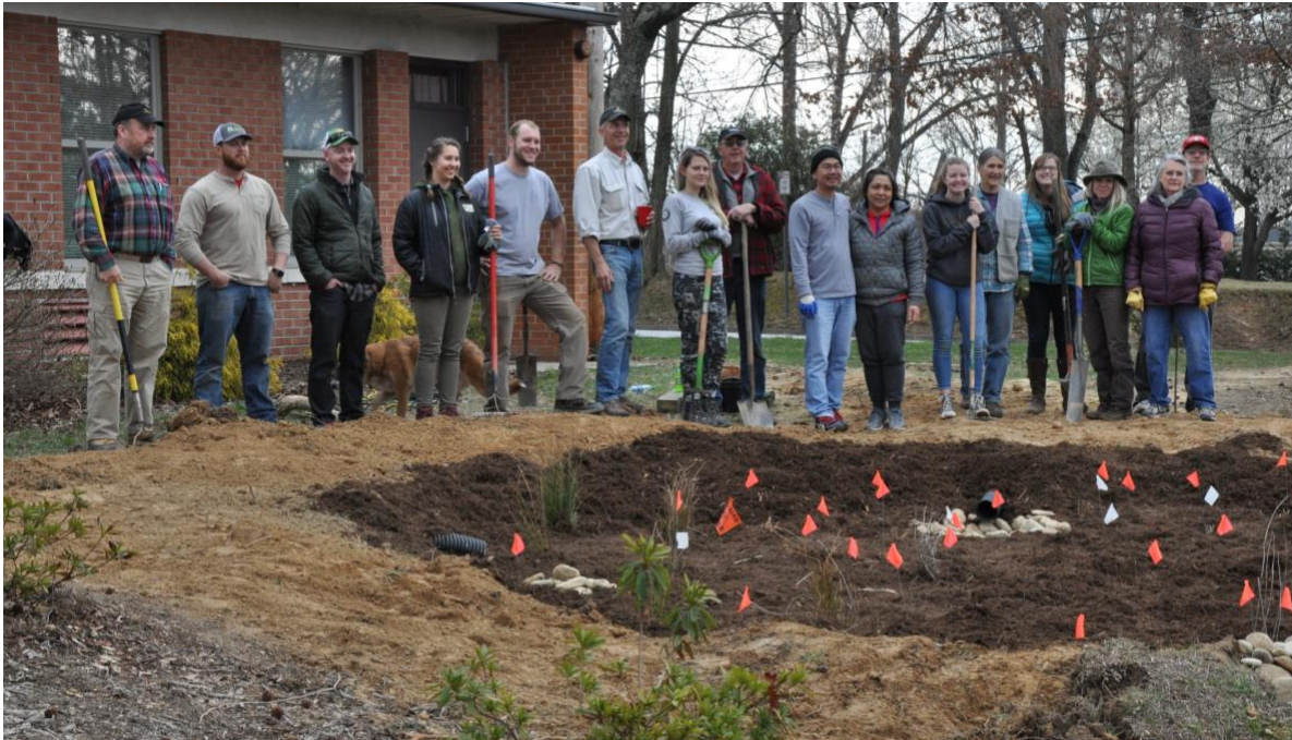
25 participants installed a rain garden using native plants at Bruce Drysdale Elementary School in March. Photo: Kim Bailey
