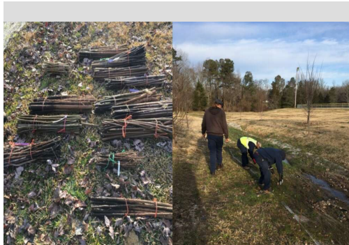
Pictures of the Carrboro Public Works staff planting live stakes as part of the riparian restoration project
